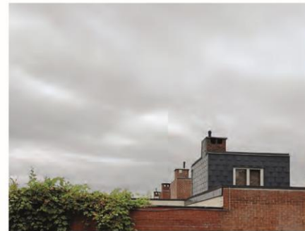
Fig 115: Shingles on a type II unit.
