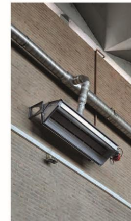
Fig 91: The flashy heaters used to warm up the church.
