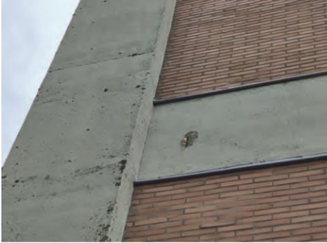
Fig 4: Spalling of concrete at the back façade, caused by the the larger volume of the corroding steel.
