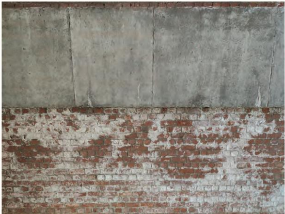
Fig 8: Effluorescence showing the present of salts due to moisture transport. Its presence is most prominent in horizontal strokes near the concrete, indicating a transport of salts from the concrete to the brickwork where it subsequently dries out.
