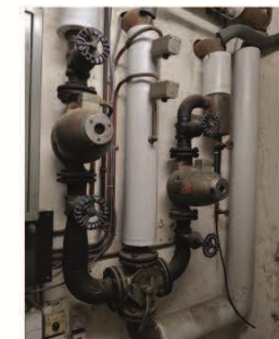
Fig 66: Outdated heating system
