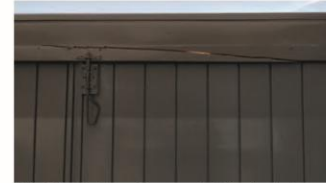
Fig 90: Tearing of the wood at the front door.
