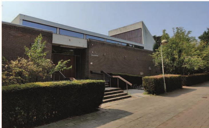
Fig 57: Northern entrance facade showing moist bricks at the top and concrete deterioration. Biological growth on the light cap.
