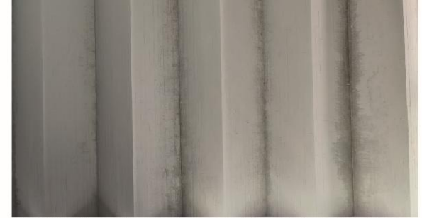
Fig 88: Possible mould formation in the pleats of the painted concrete roof structure
