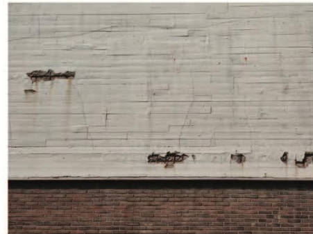
Fig 56: Flaking, scaling and cracking due to concrete carbonation. The corrosion of reinforcement leaving stains.
