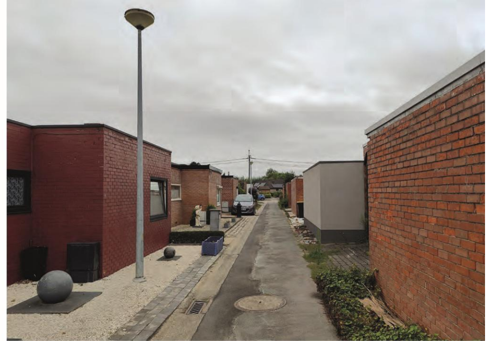
Fig 114: Low-traffic street showing the multiple different new facade finishings and roofs. Some of the bricks of the original façades are showing deterioration.
