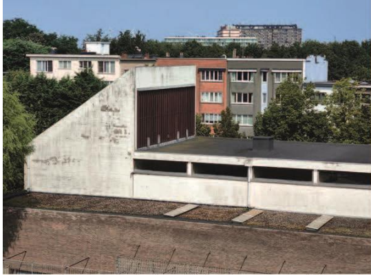
Fig 55: Chapel exterior showing exfoliation of vapour proof paintlayer. Moist bricks due to absence of a sufficient roof overhang.
