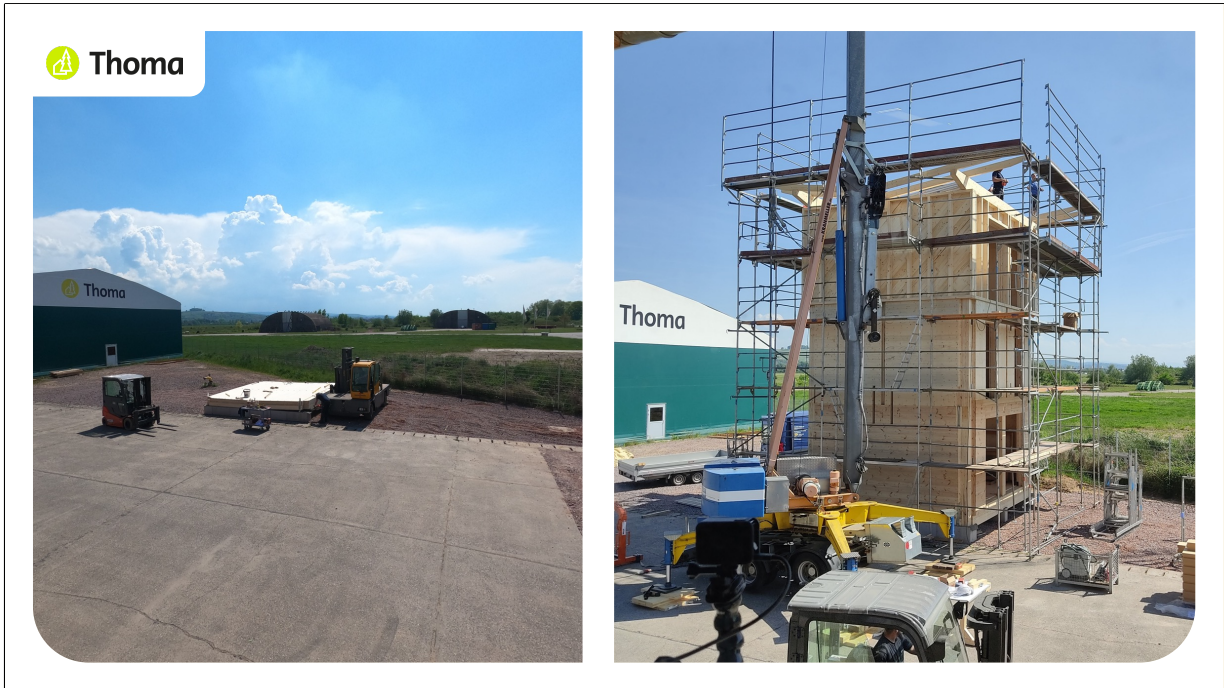
From floor slab to finished 3-storey building in 2 days! There was no screwing required during assembly.
